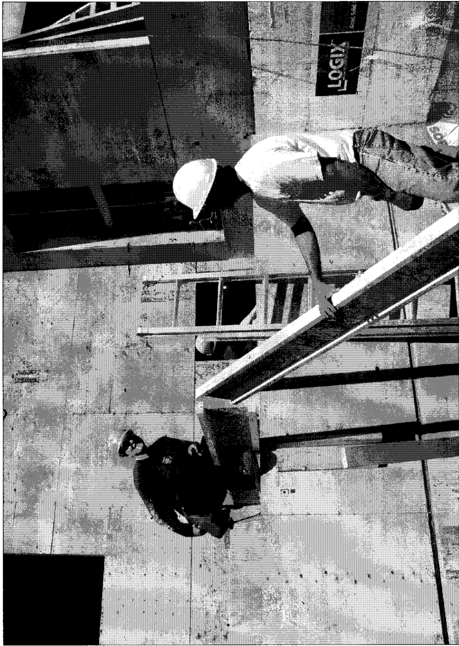
Student carpenters work on Okanagan College's first residential construction project. Melissa Jameson/Times Review
