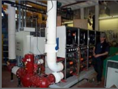
Heat Recovery Chiller - Doors Removed
